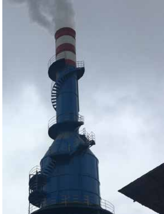
喷淋设施及排气筒
